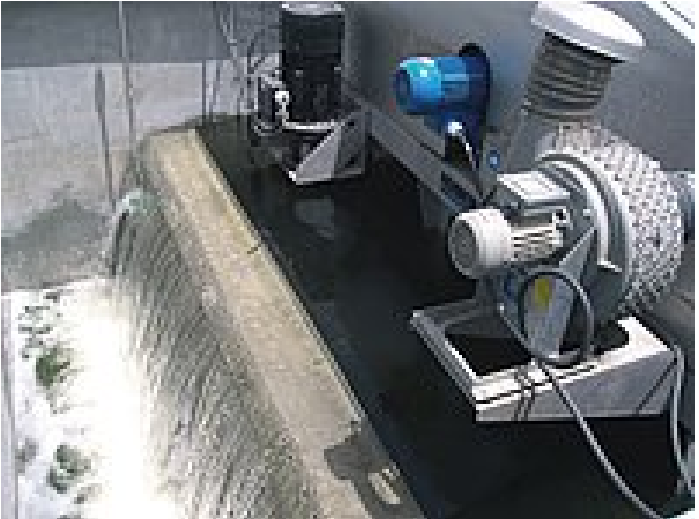
Effluent from our RoDisc® 20 micro-screens
