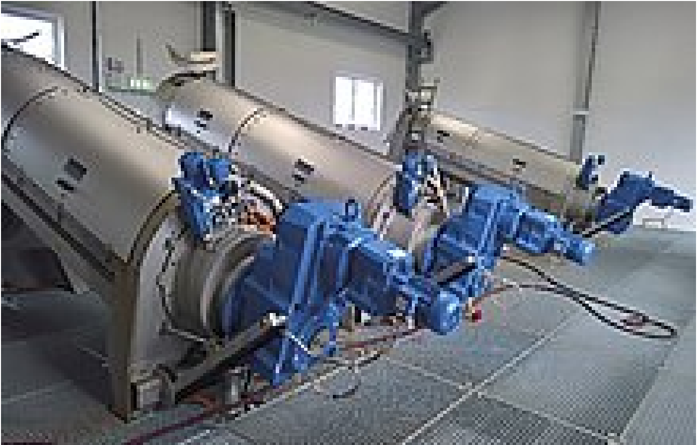
Three HUBER Screw Press Q-PRESS® 620 (two units dewater surplus sludge, 1 unit dewateres flotote sludge)
