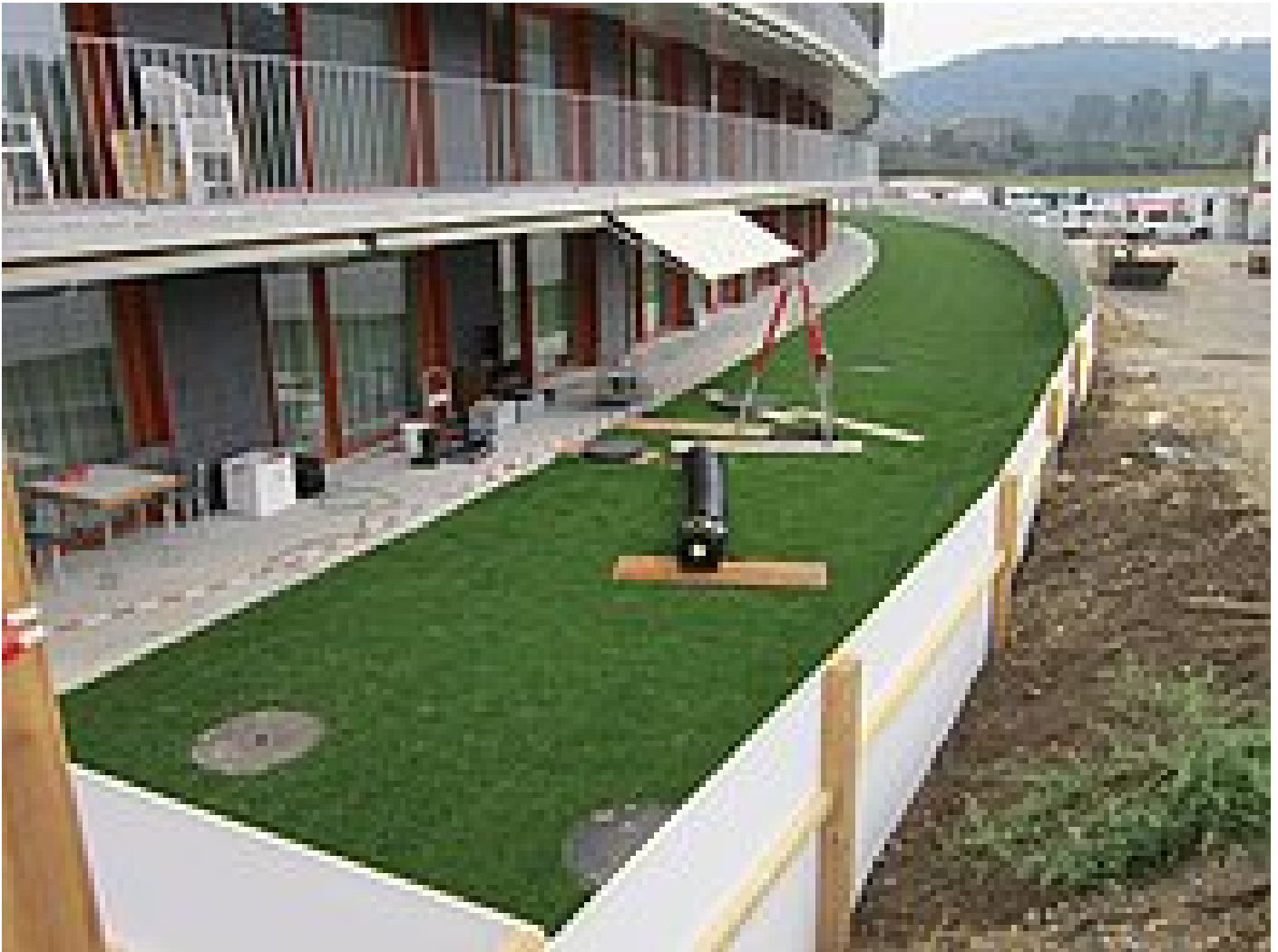
Figure 1: Old-age home Hofmatt in Münchenstein after the first stage of modernisation with the entrance to the wastewater shaft in the garden
