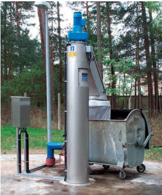
Screenings discharge into a bagger
