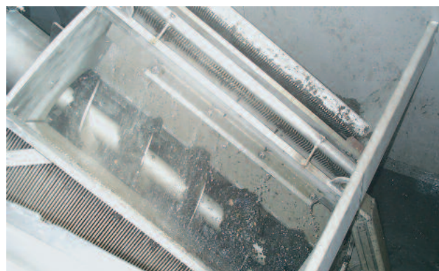
Debris and other coarse solids are retained in the screen basket; rake tines fully penetrate the slots between its bars thus guaranteeing positive cleansing
