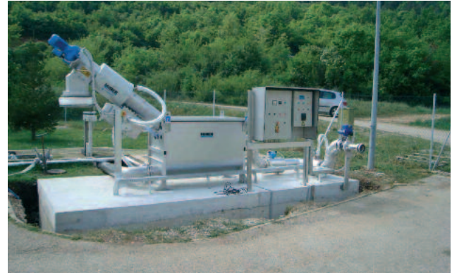
ROTAMAT® Ro 3.1 Septage Receiving Station at the plant entrance
