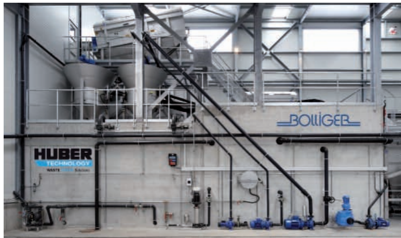
Smart pump technology arrangement to ensure easy access for maintenance
