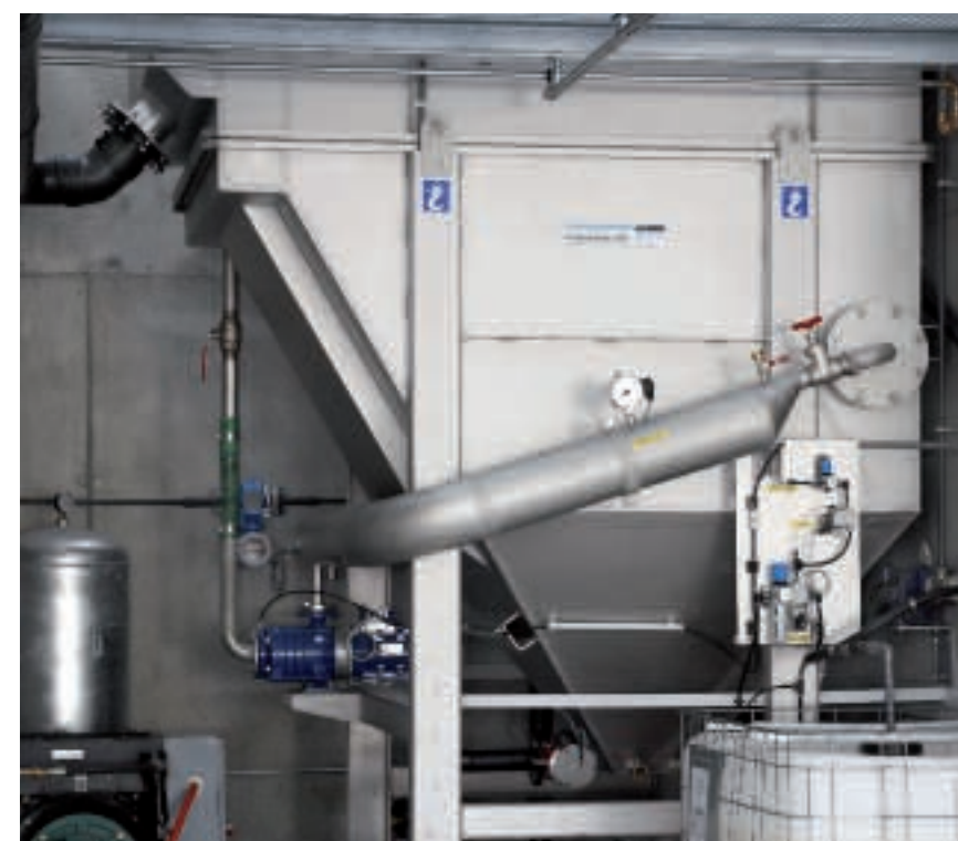
HUBER Dissolved Air Flotation Plant for process water treatment
