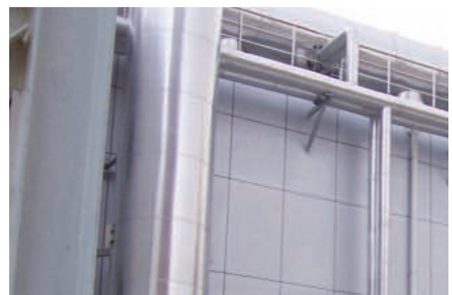
Condensation stage of line 1
