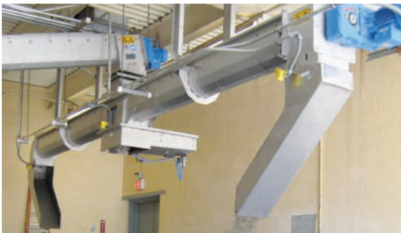
Distribution screw for dewatered sludge, Kennebunk
