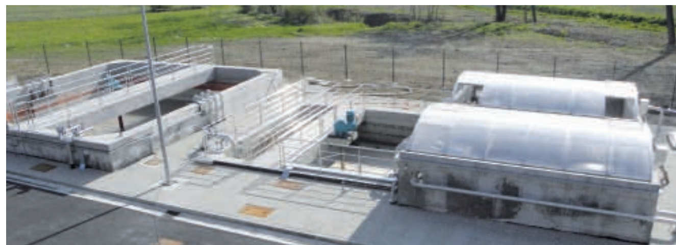
Mixing and balancing tank, bio-tank and HUBER MBR system
