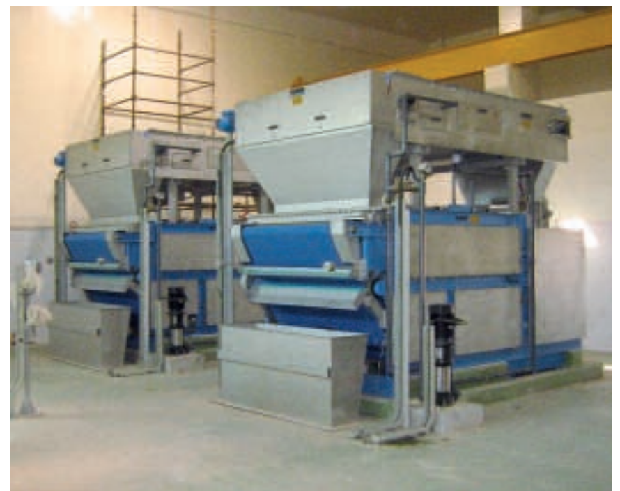
Two lines of the BS Combi belt filter presses with belt thickeners mounted on top before start-up
