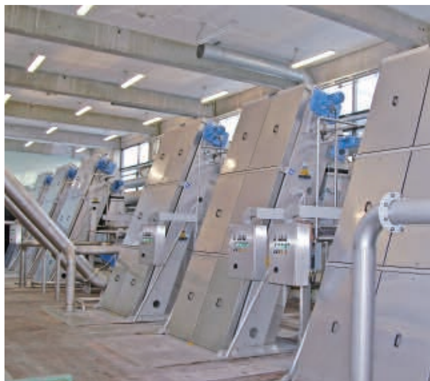
HUBER Belt Screen EscaMax® on WWTP Damhusaen
