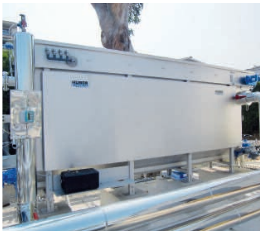
A HUBER Heat Exchanger RoWin installation on the Côte d'Azur
