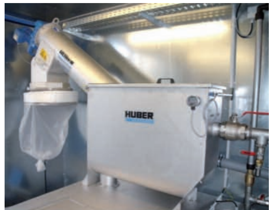
Mechanical preliminary screen (HUBER ROTAMAT® Micro Strainer Ro 9)
