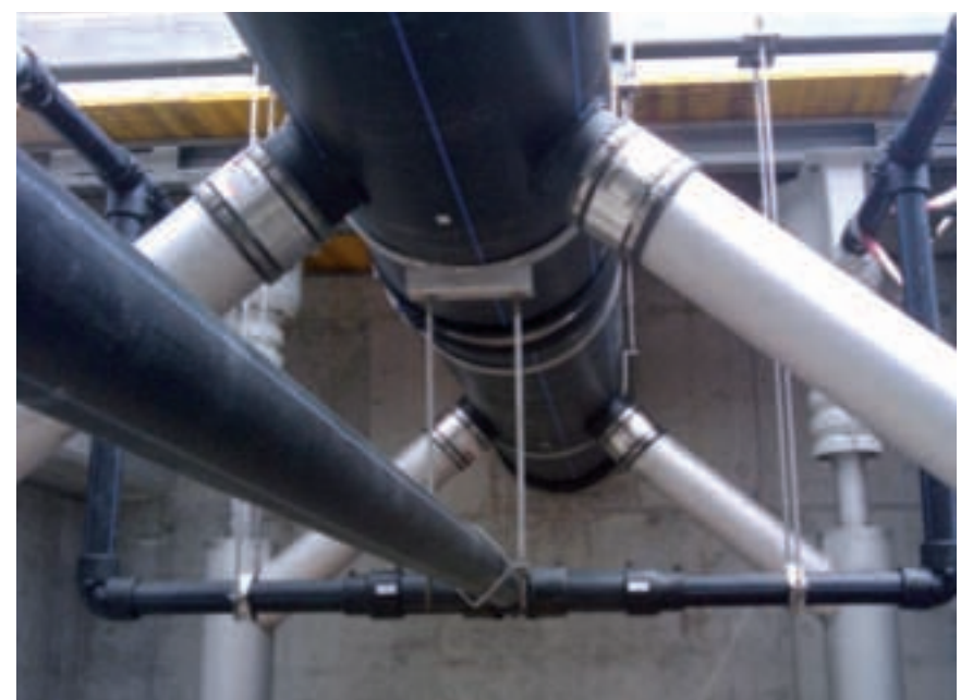
Built-in components of CFSF 50 C – interaction of different materials with corrosive waters
