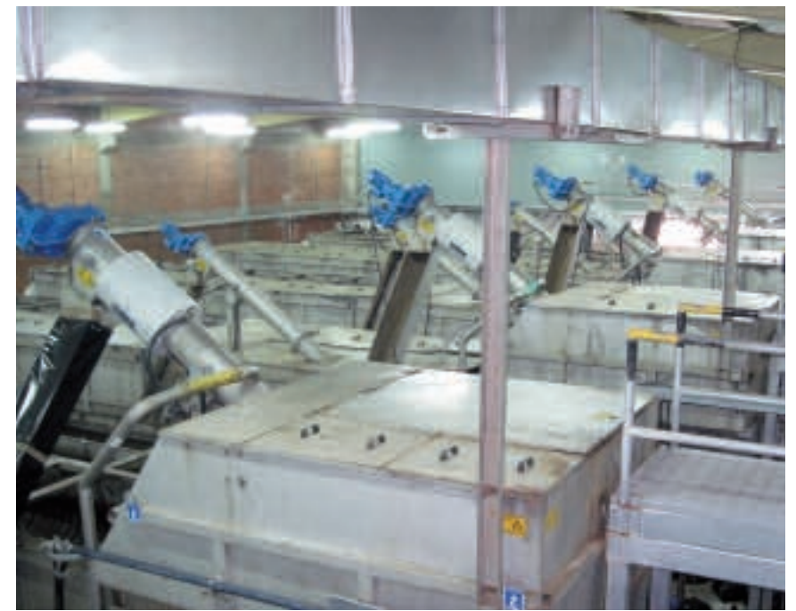
Six wastewater treatment lines in the inlet to WWTP Coquimbo
