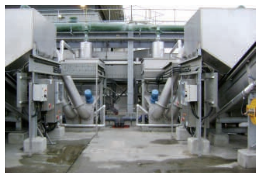
HUBER Wash Press WAP SL, Dublin Bay (UK)
