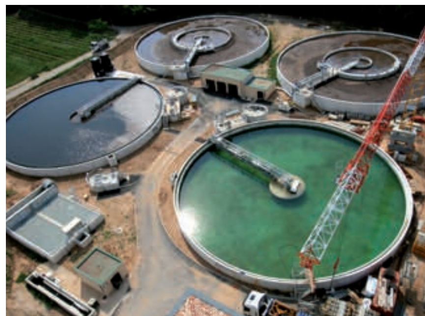
Size comparison: Sandfilter with 20 filters (bottom left) – total WWTP for approx. 150,000 PE
