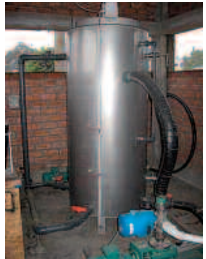
Biogas Reactor in Carrapongo
