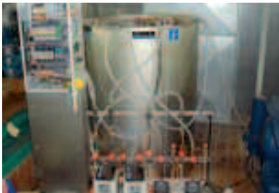
Membrane Bio-Reactor Test Plant
