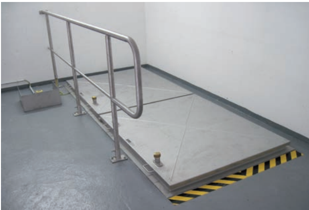
SD 1.2 Two-part manhole cover for stairway, railing as antiffall guard
