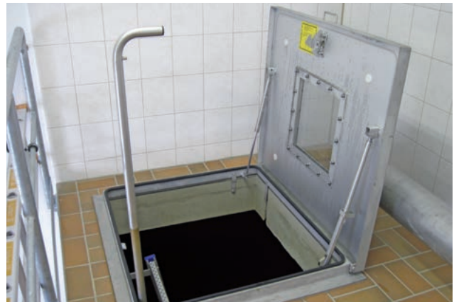
SD 1 Manhole cover SD 1, rectangular, with window
