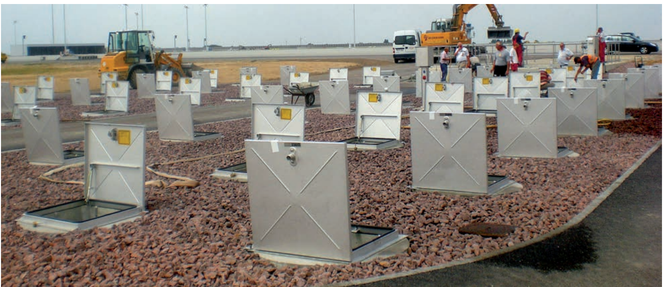
SD 1 Manhole covers, airport Leipzig
