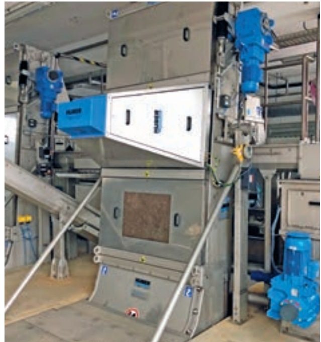
Figure 1: HUBER Safety Vision installed on a HUBER Multi-Rake Bar Screen RakeMax®.
