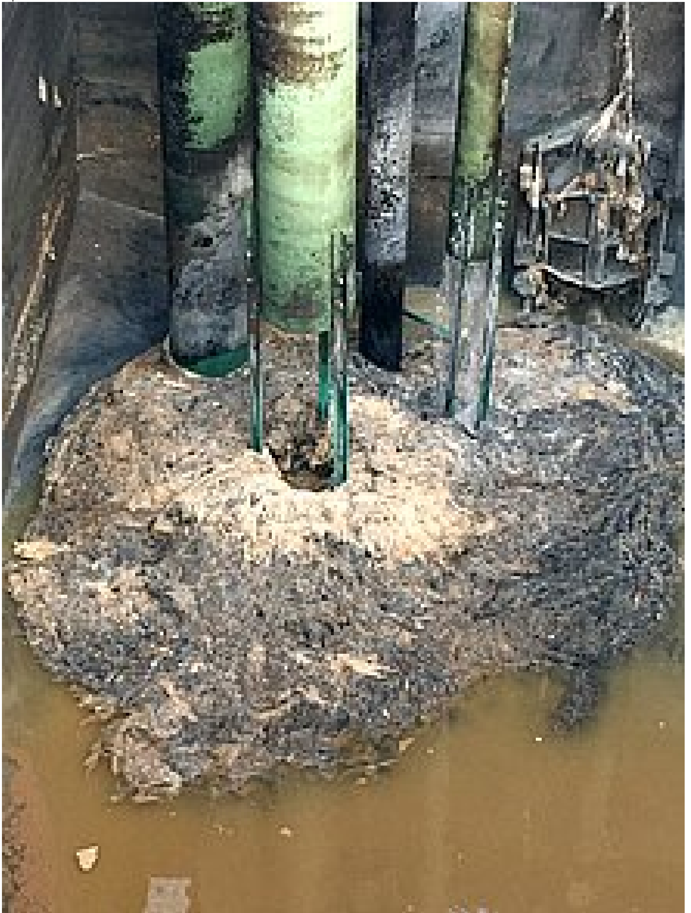
Screenings build up in balance tank – before screens were fitted
