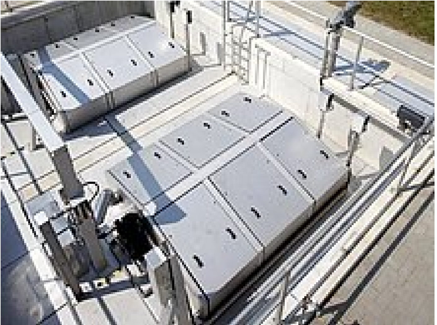
HUBER RoDisc® Rotary Mesh Screens in a concrete tank
