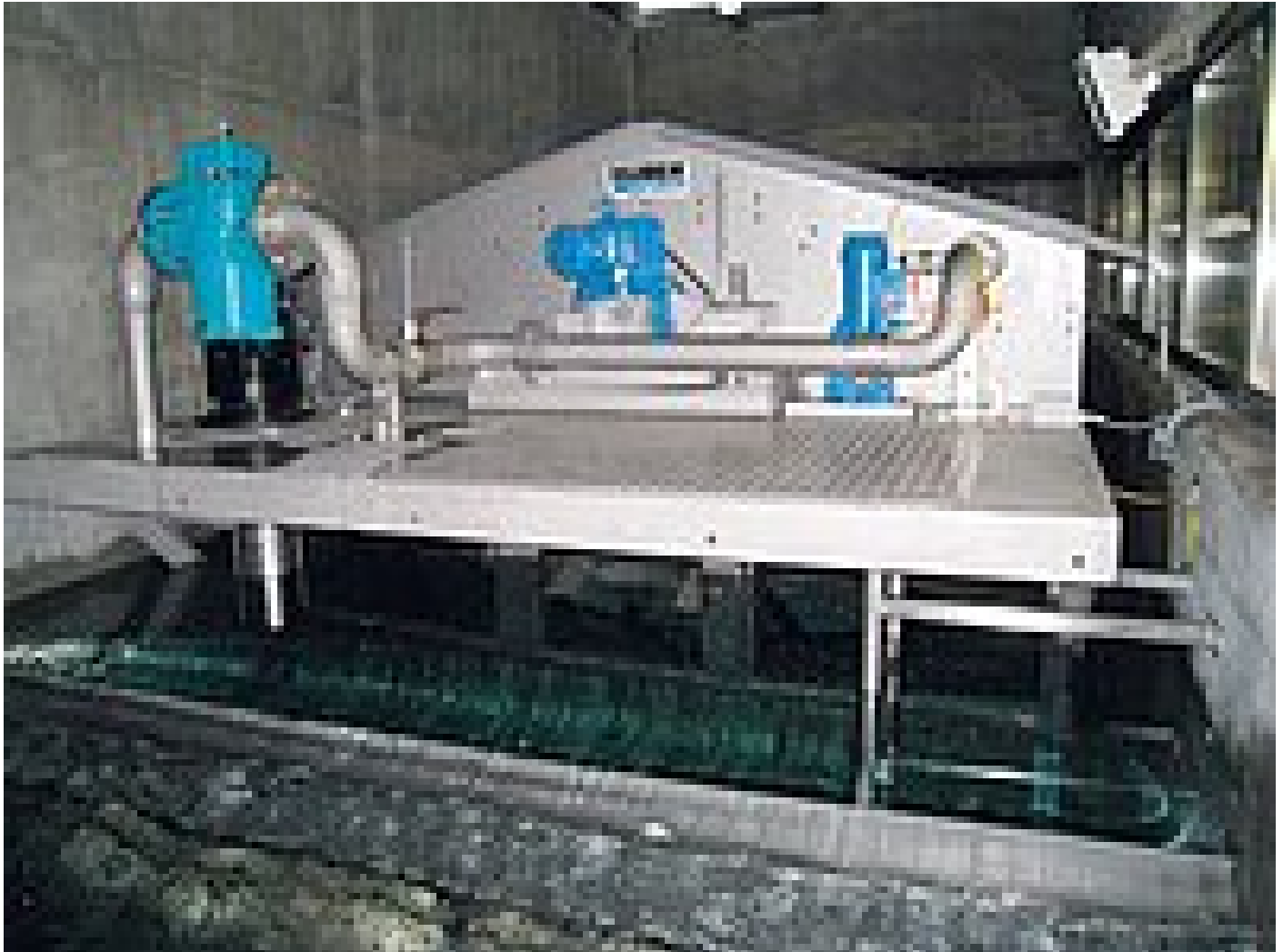
RoDisc® Rotary Mesh Screen installed in the inlet structure from where a 10 km long pipeline runs to the water works
