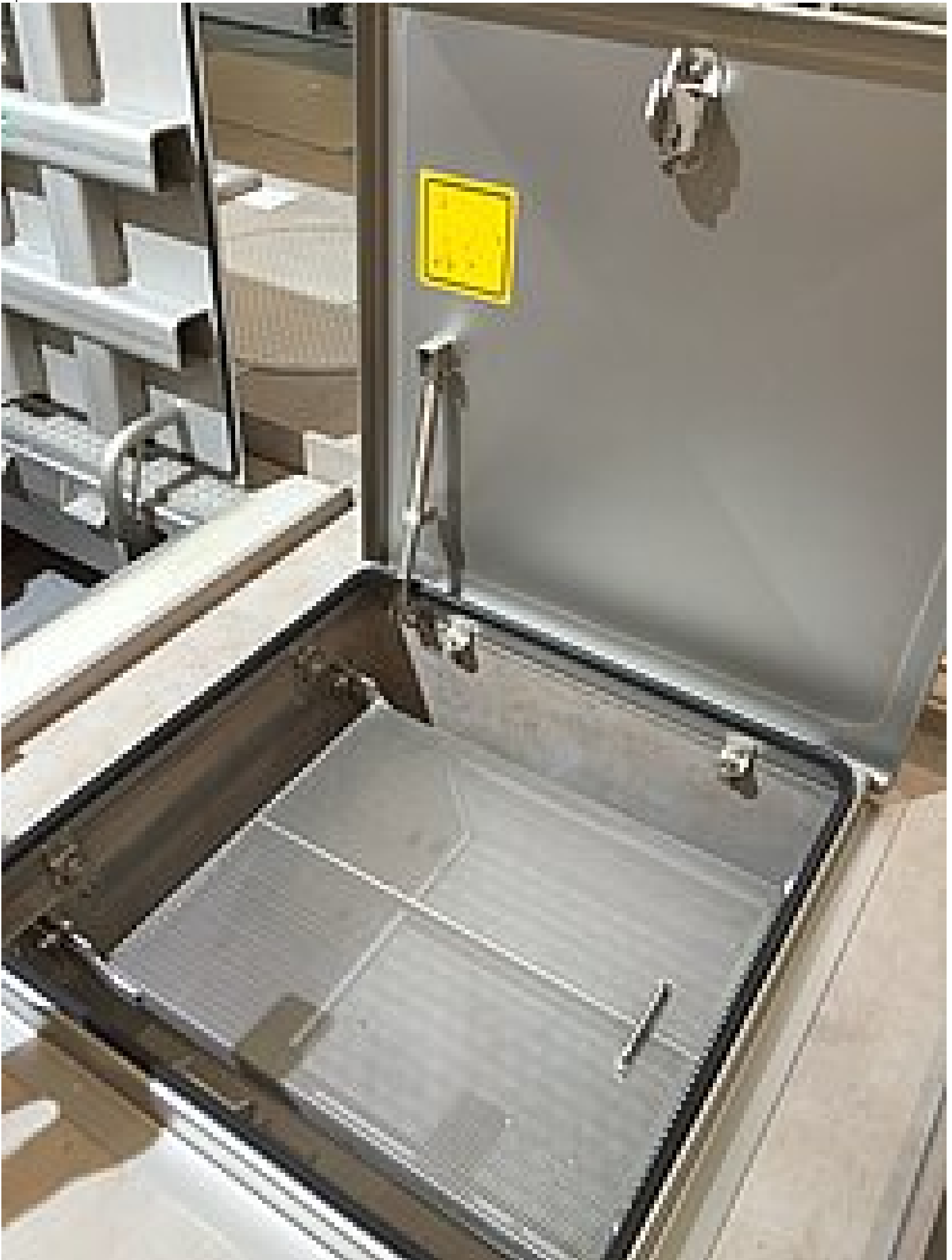
Manhole cover with antifall guard – closed
